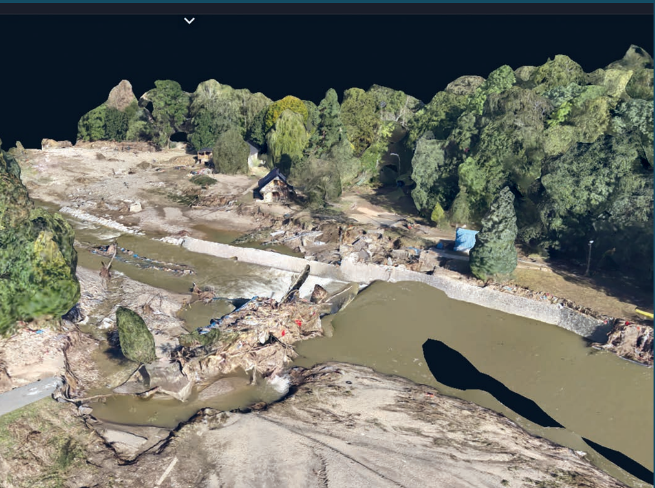
Water sill/jam on the Głuchołaska Biała River. Measurable 3D model created after the passage of a destructive flood wave. Made via BSP due the very difficult access to the site by land. At the same time, the model allows a numerical and quantitative assessment of the restoration of access roads to the site. In addition, it provides information on the amount of loose material needed to restore the river to its natural channel.
